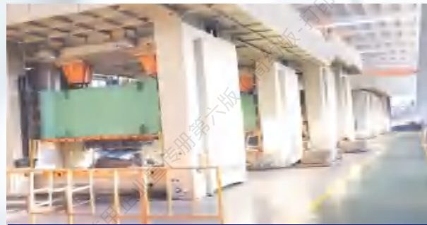
冲压-400T-2000T冲压生产线两条 Two stamping production lines for stamping -400T-2000T
